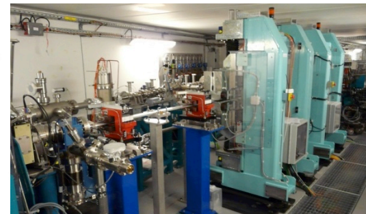
3 magnet chicane of a few mrad, to adjust the photon beam at center of the first beamline mirror.
