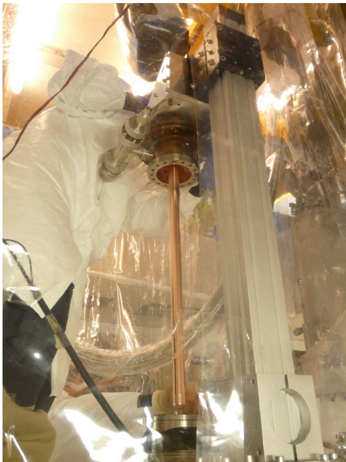
3rd RF power coupler installed in January 2016
